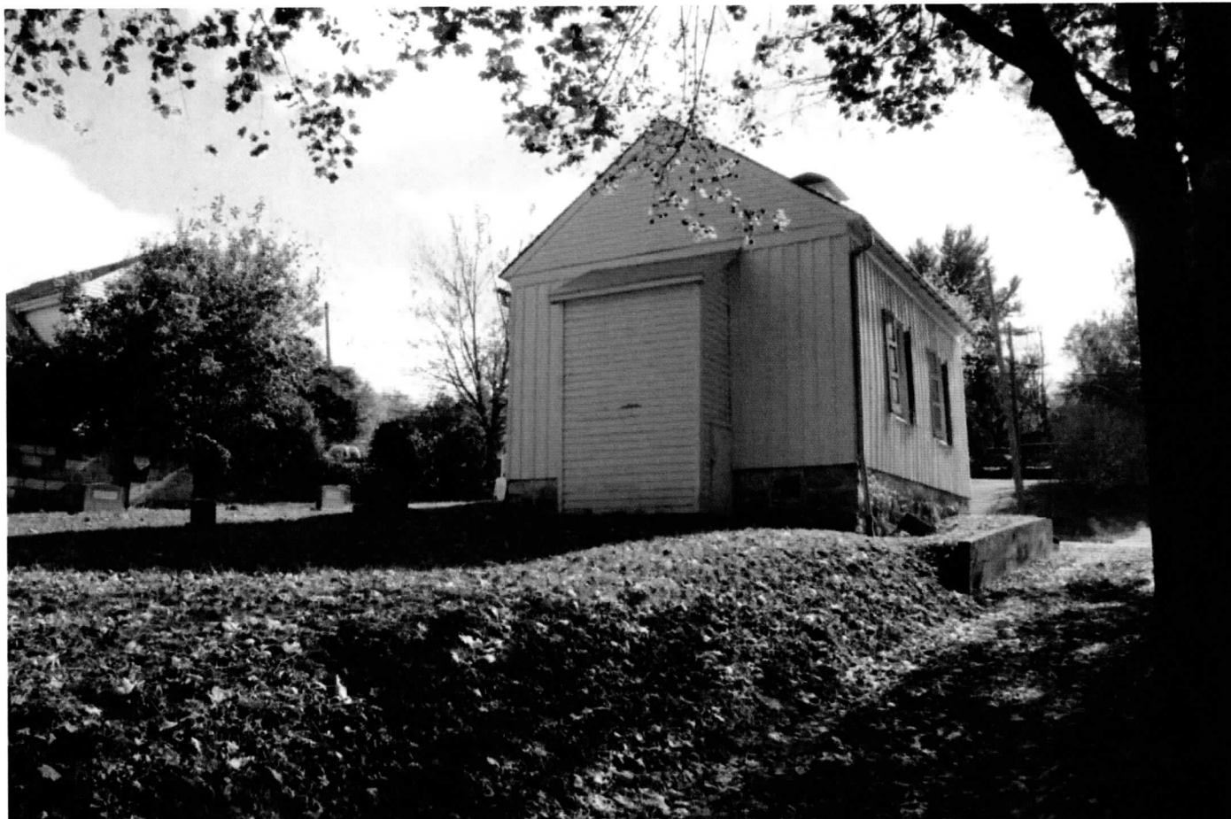
4 of 10 North and west elevations of church/school, looking southeast from west alley.
