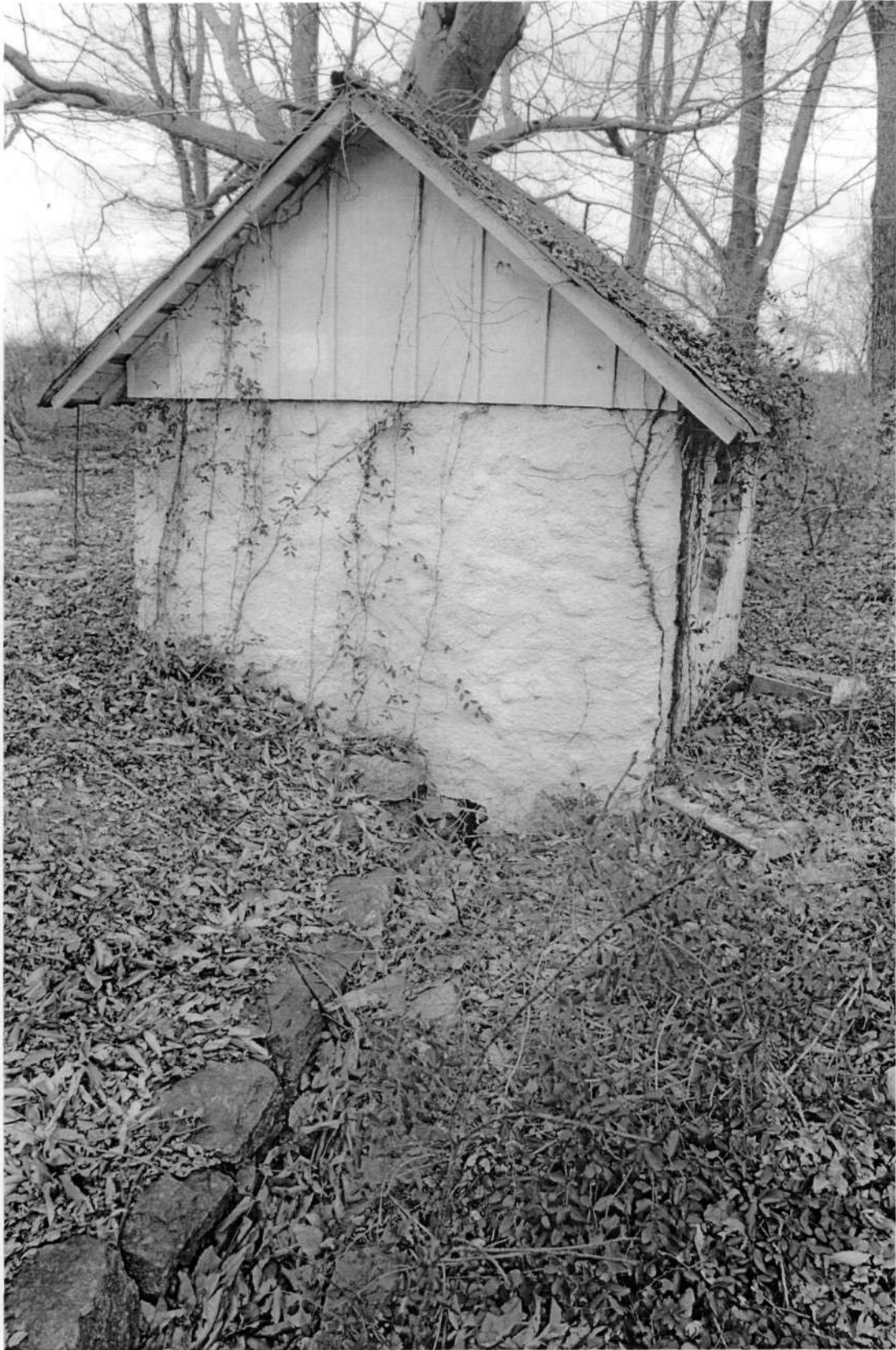
HO-929 Dasher Farm Cradlerock Farm Court Springhouse, south elevation Ken Short, December 2006 3/4
