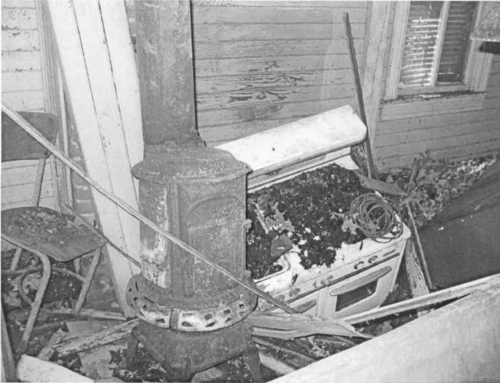
First floor interior, facing south. Stove falling through floor.
