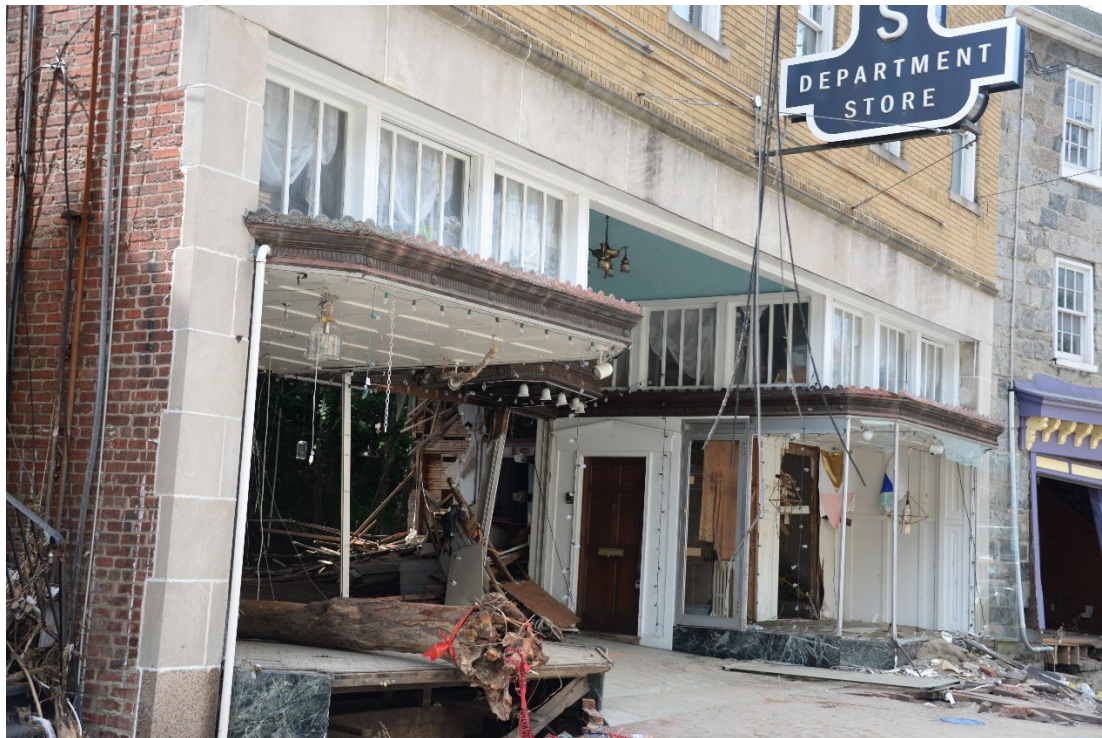
Photo 10 of 15: North elevation, storefront following 2016 flood. 8/10/2016
