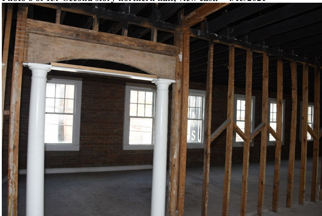
Photo 7 of 15: Second story doorway with moved columns at west end of partition wall, view north. 4/15/2021
