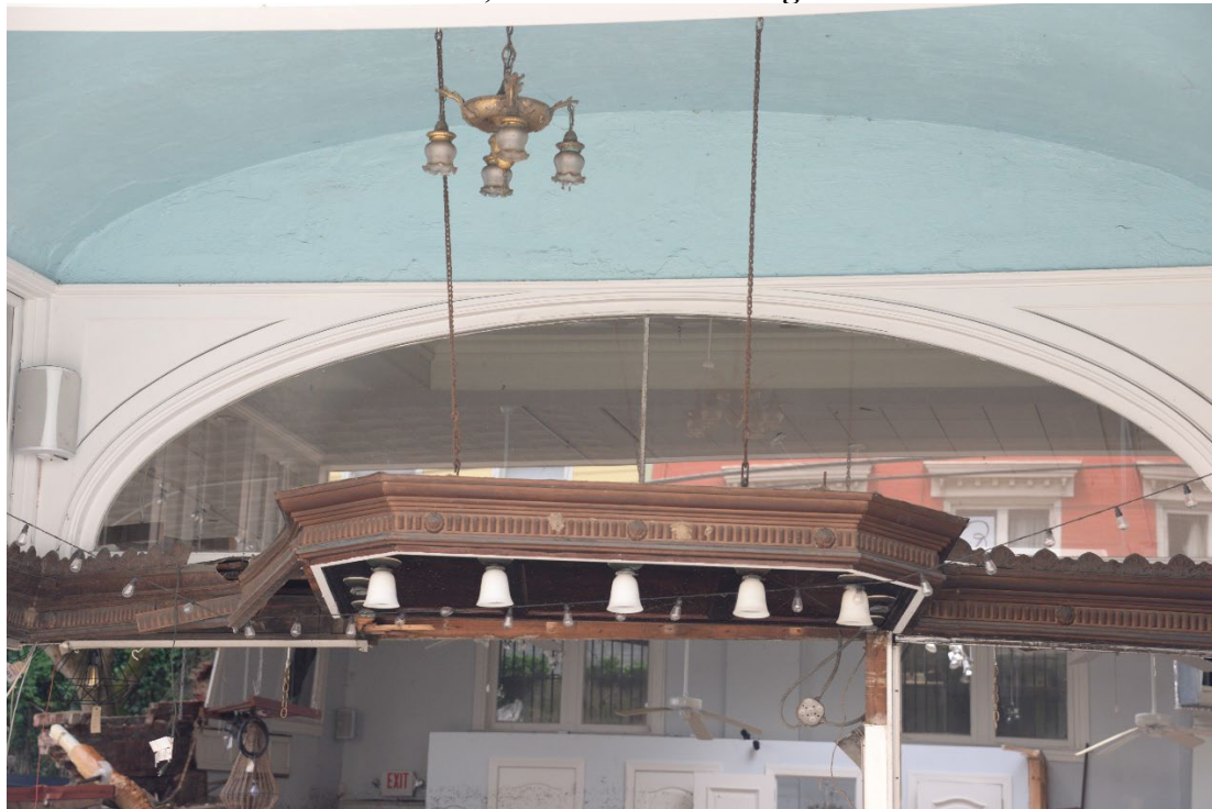
Photo 11 of 15: North elevation, door hood following 2016 flood. 8/10/2016
