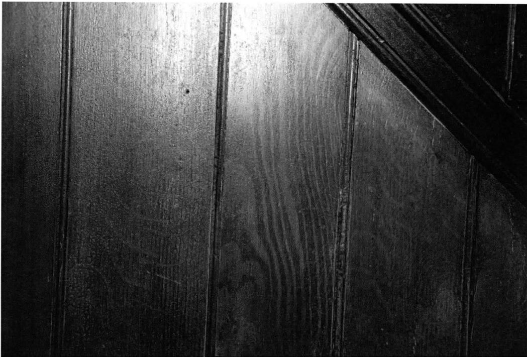
Photo 4 of 16: First-story passage, graining on boards under stair. 4/10/2017
