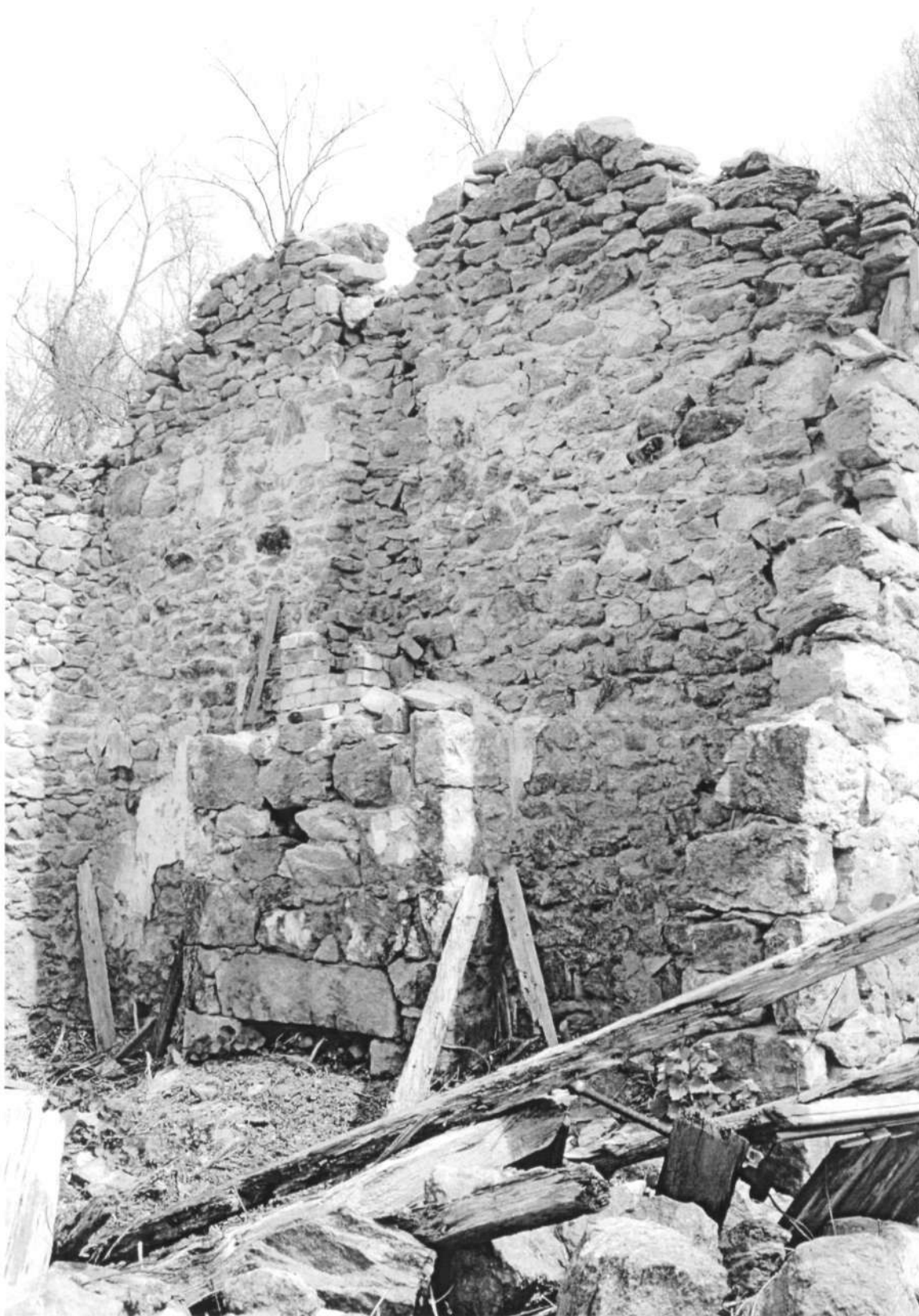
HO-411 Woodlawn Slave Quarter 9254 Old Annapolis Road West section, interior, east elevation Ken Short, April 2006 5/14
