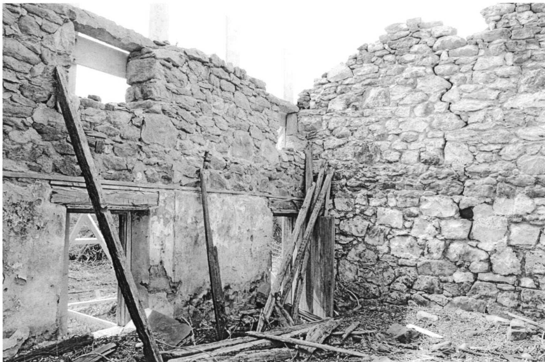
HO-411 Woodlawn Slave Quarter 9254 Old Annapolis Road East section interior, south & west elevations Ken Short, April 2006 7/14
