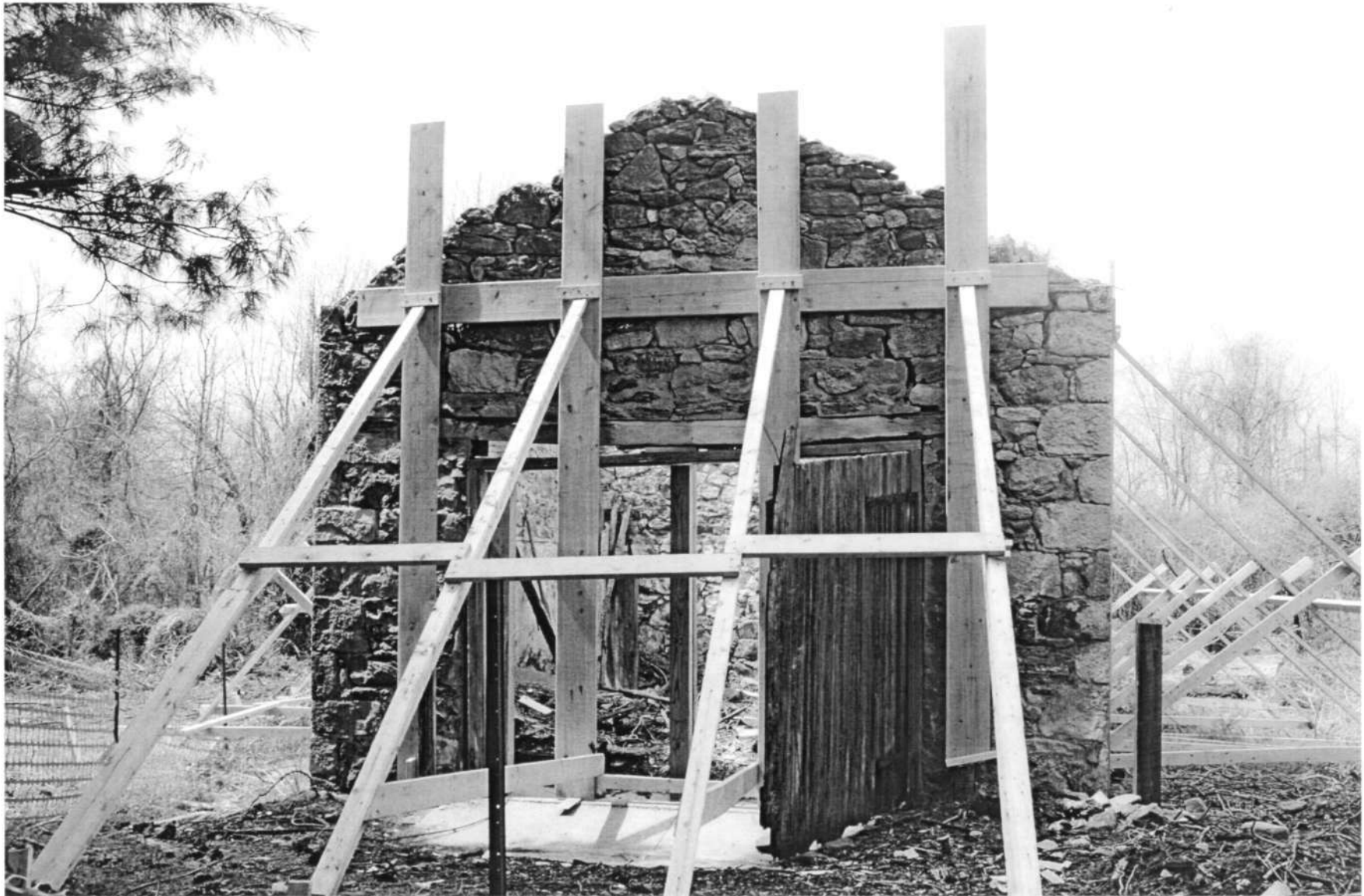
HO-411 Woodlawn Slave Quarter 9254 Old Annapolis Road East elevation Ken Short, April 2006 4/14
