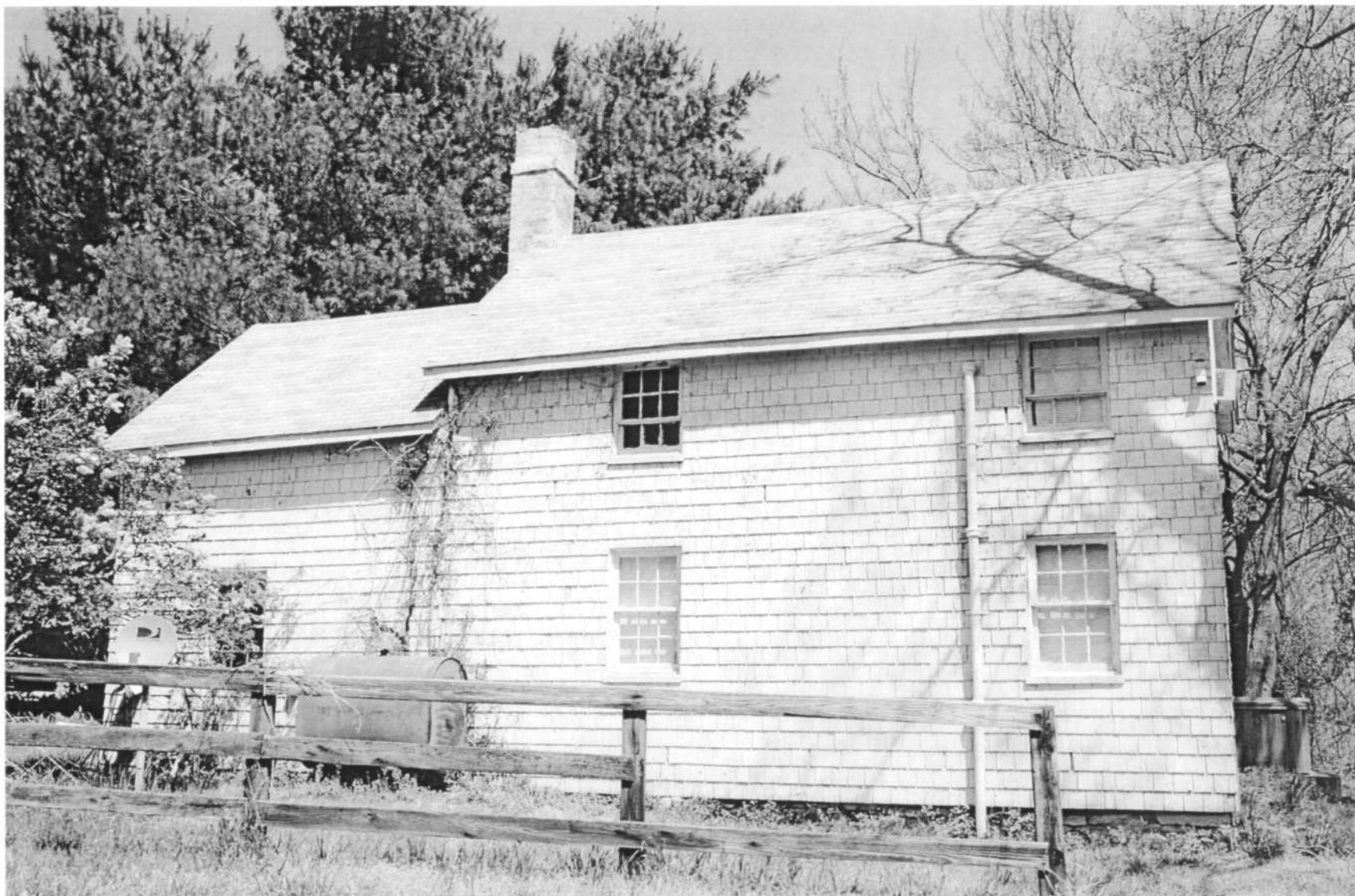
HO-411 Woodlawn Slave Quarter 9254 Old Annapolis Road Cottage, west elevation Ken Short, April 2006 9/14
