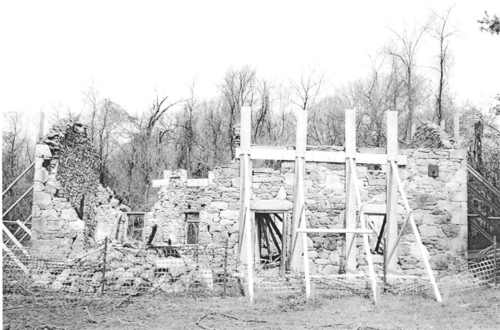
HO-411 Woodlawn Slave Quarter 9254 Old Annapolis Road south elevation Ken Short, April 2006 1/14
