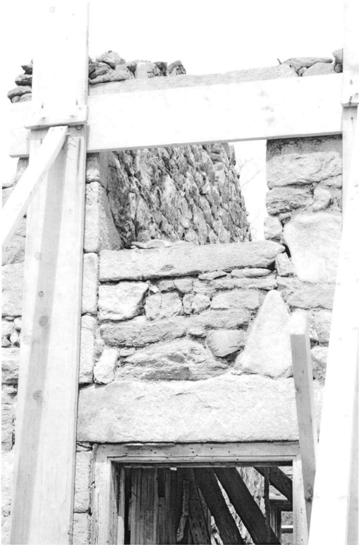
HO-411 Woodlawn Slave Quarter 9254 Old Annapolis Road south elevation, joint between east & west sections Ken Short, April 2006 2/14
