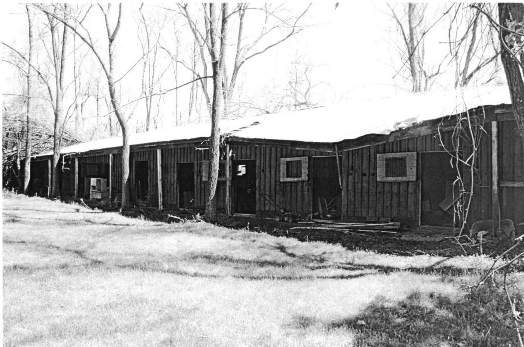
HO-411 Woodlawn Slave Quarter 9254 Old Annapolis Road Stable, north elevation Ken Short, April 2006 12/14
