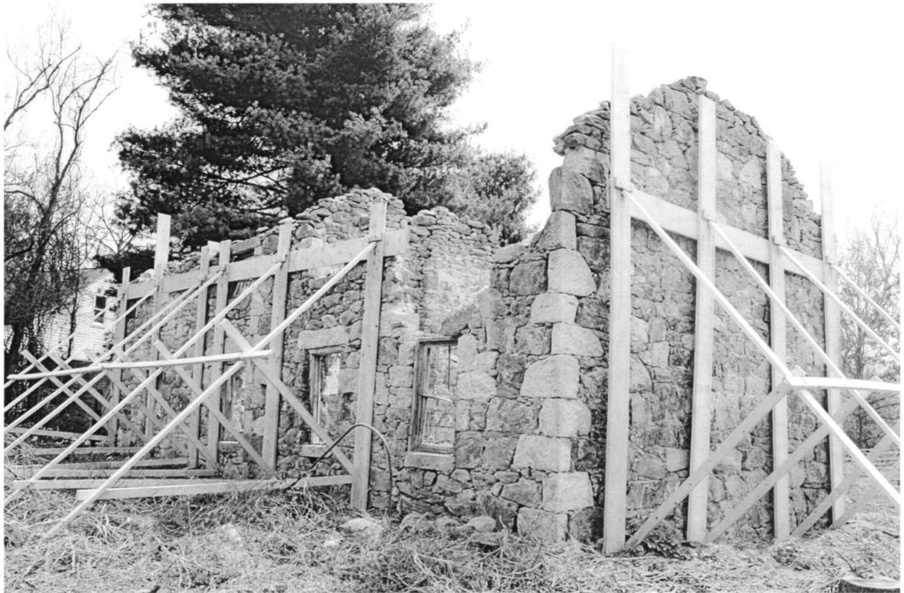
HO-411 Woodlawn Slave Quarter 9254 Old Annapolis Road North & west elevations Ken Short, April 2006 3/14
