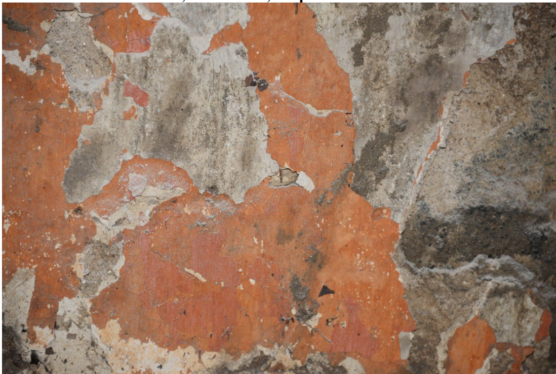
Photo 16 of 19: Basement, main block, traces of plaster and paint on east wall. 2/24/2017
