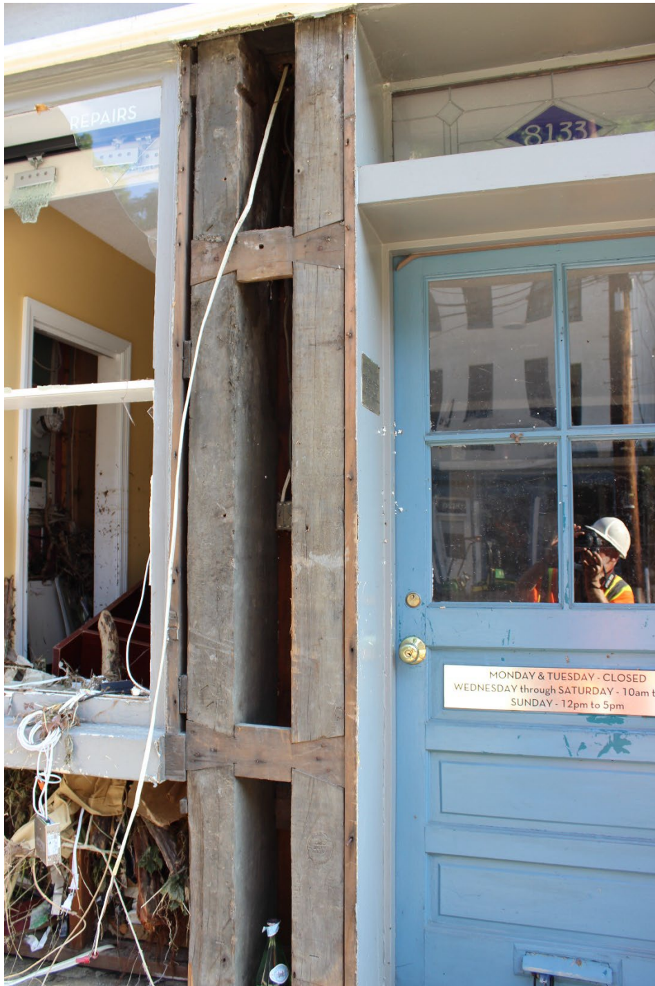
Photo 19 of 19: North elevation showing post construction exposed after 2016 flood. 8/2/2016
