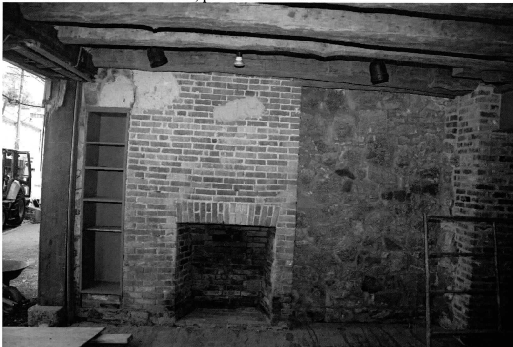
Photo 3 of 10: First story, east elevation. 9/15/2016
