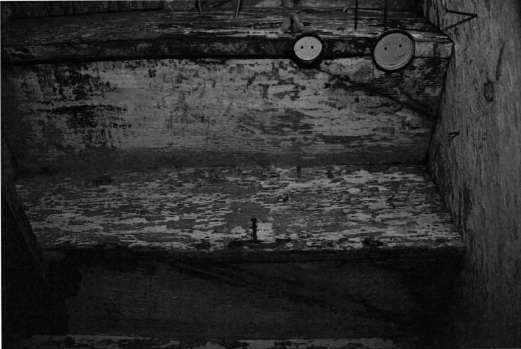
Photo 13 of 19: 8329 – South room, bottom of first story stair treads with seams showing reused winders. 8/2/2021
