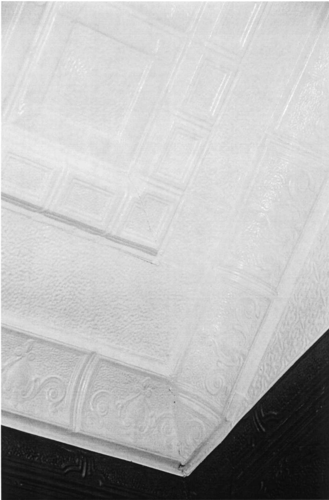
HO-0276 Mt. Gregory United Methodist Church 2325 Maryland Route 97, Interior cornice and ceiling Ken Short, March 2006 9/11
