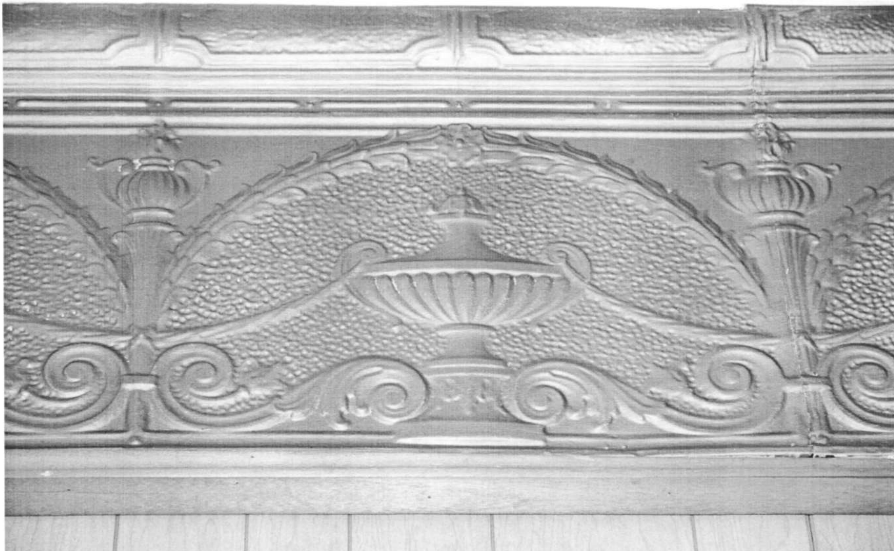
HO-0276 Mt. Gregory United Methodist Church 2325 Maryland Route 97, Interior, frieze Ken Short, March 2006 8/11
