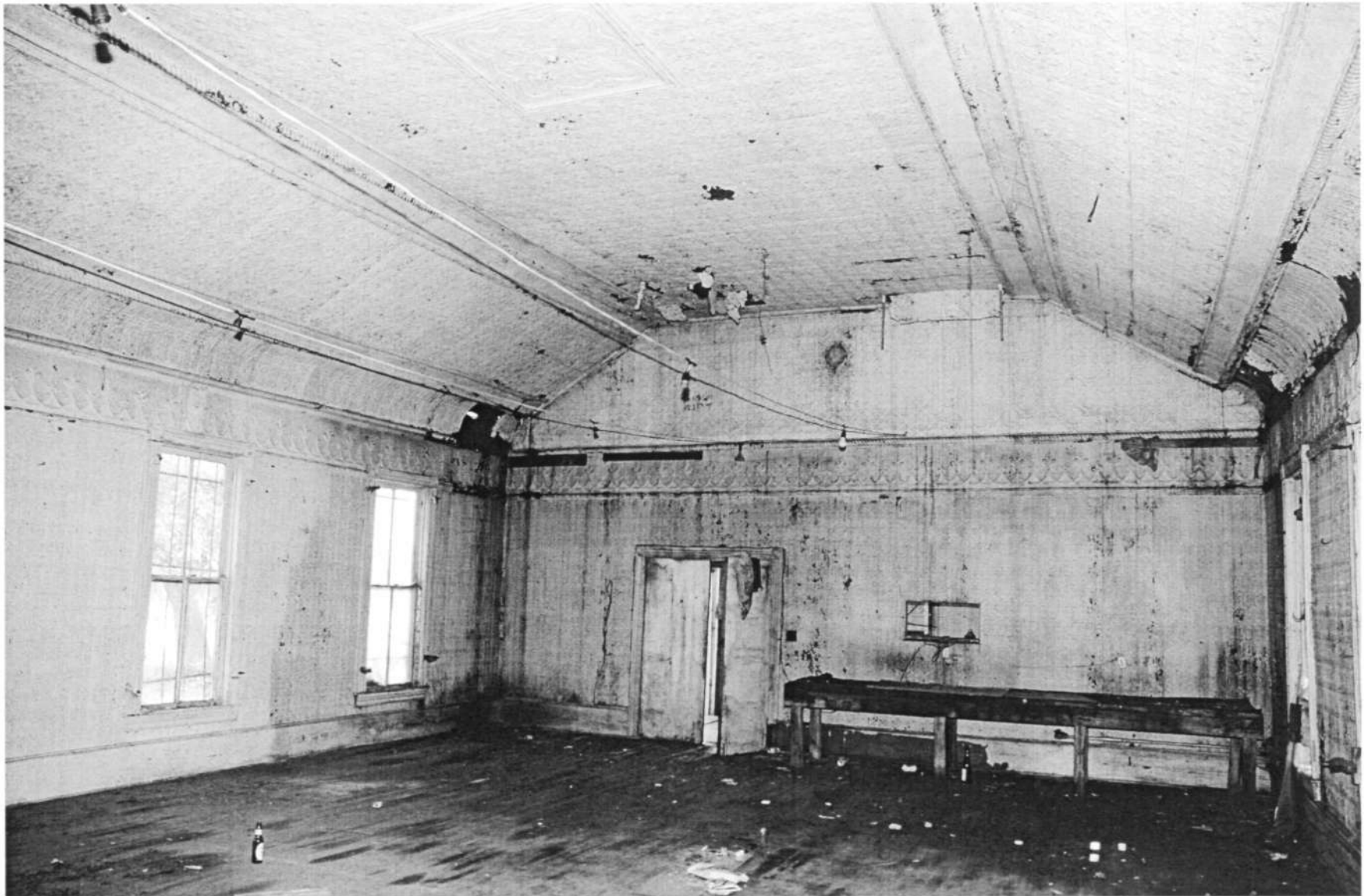
HO-259 International Order of Good Templars Hall 15905 Union Chapel Road Interior, vw. northwest Ken Short, August 2006 5/13
