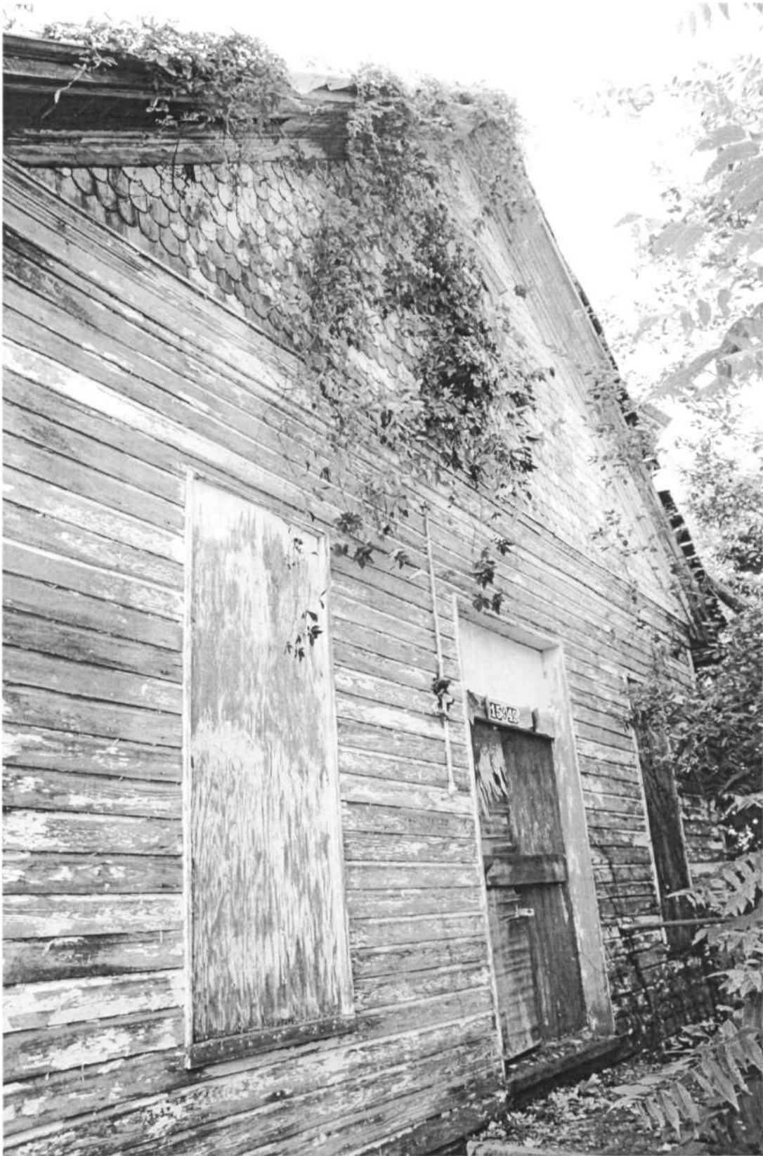
HO-259 International Order of Good Templars Hall 15905 Union Chapel Road North elevation Ken Short, August 2006 2/13
