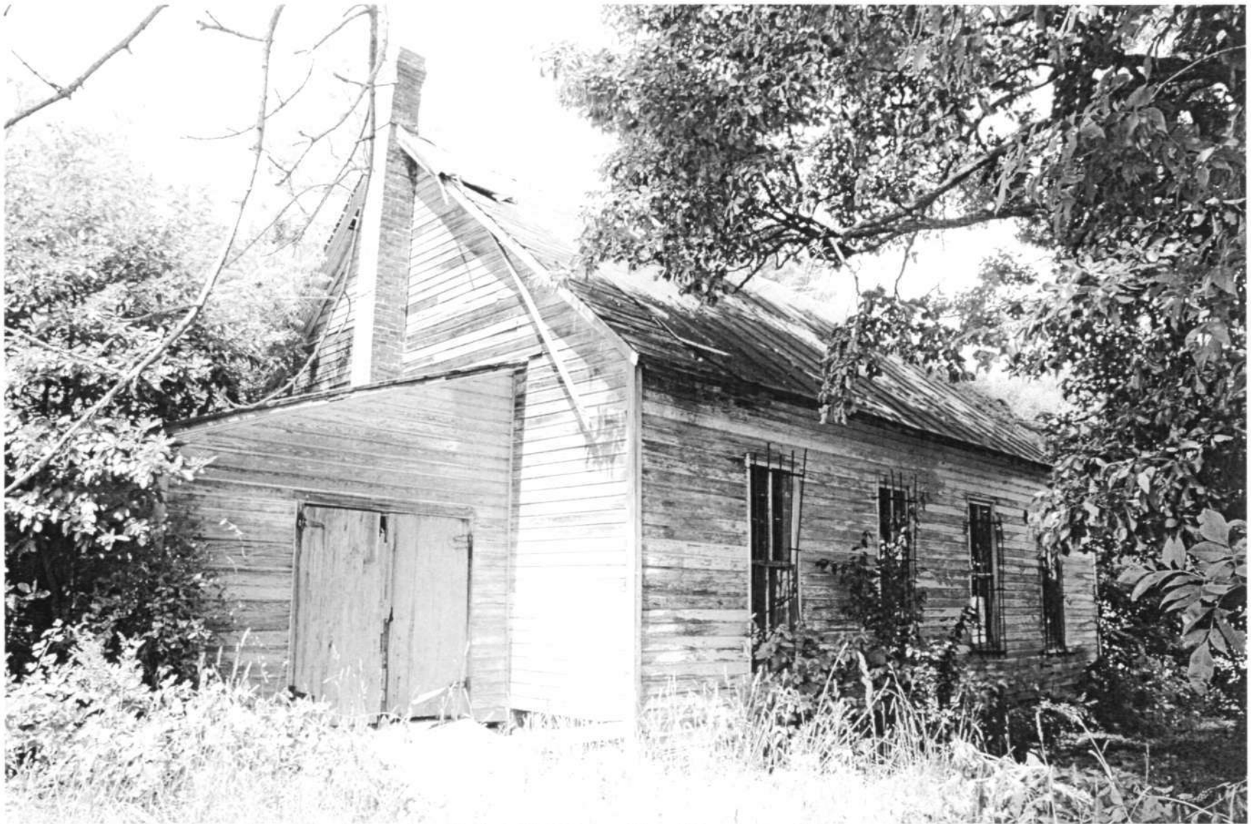
HO-259 International Order of Good Templars Hall 15905 Union Chapel Road South & east elevations Ken Short, August 2006 4/13
