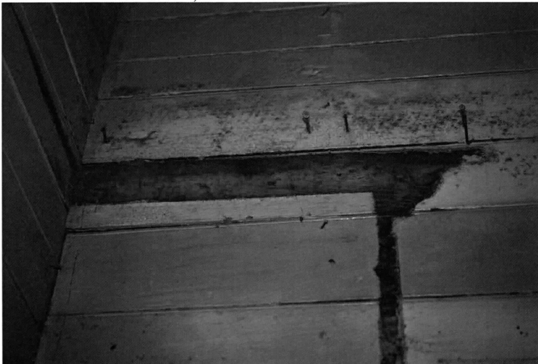
Photo 4 of 13: Store interior, south elevation, detail of shelf cornice ghost at east end. 5/14/2020
