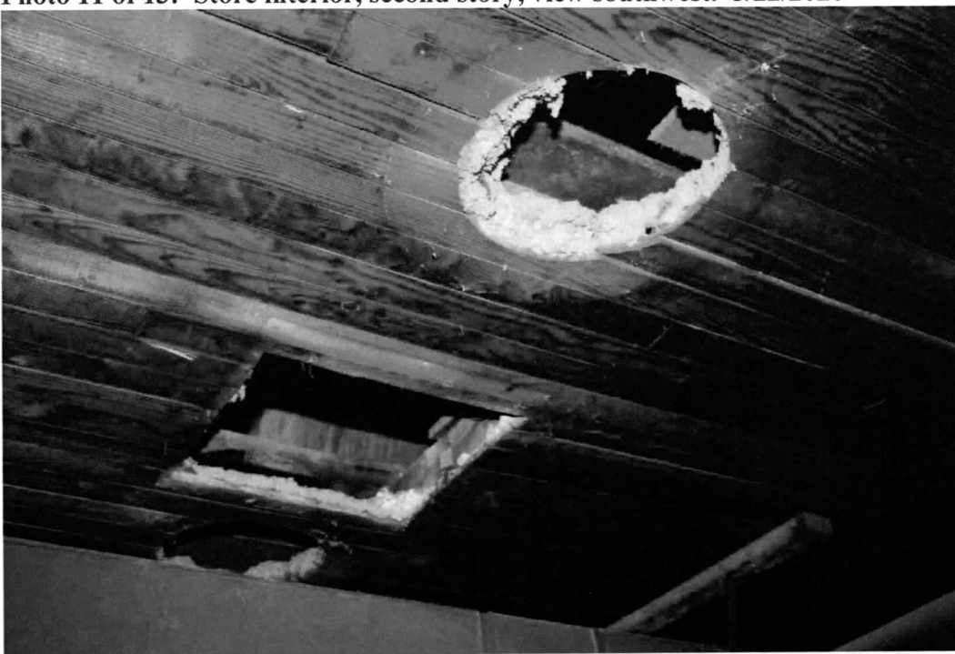
Photo 12 of 13: Store interior, second story, holes for vents in ceiling. 5/22/2020
