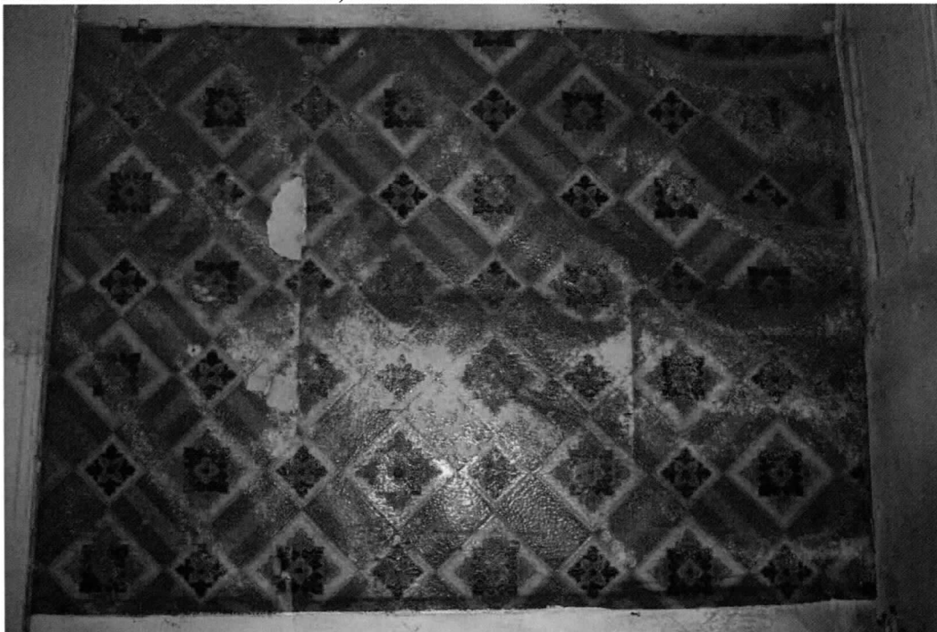
Photo 6 of 13: Store interior, linoleum wall covering on west elevation, at north end. 5/14/2020
