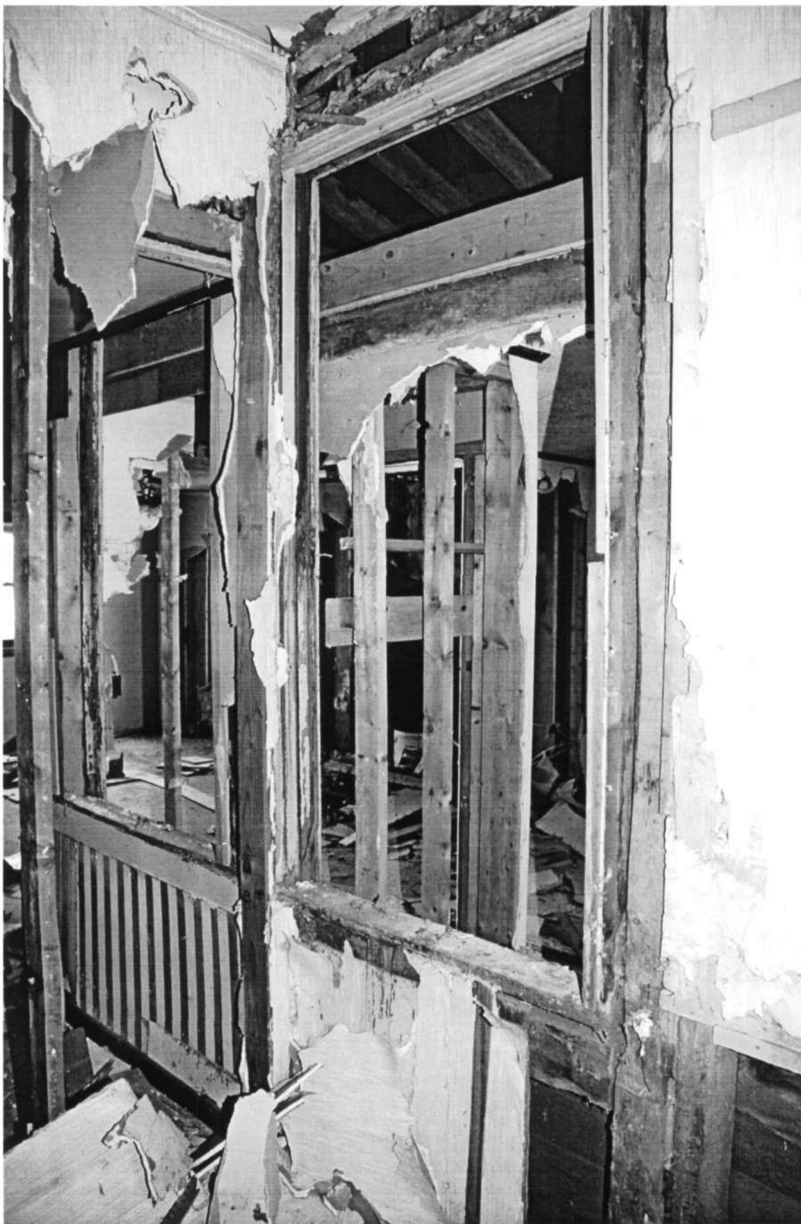
HO-0253 Old Florence School 3055 Florence Road, Original window openings in northwest wall, from southeast Ken Short, April 2006 7/9
