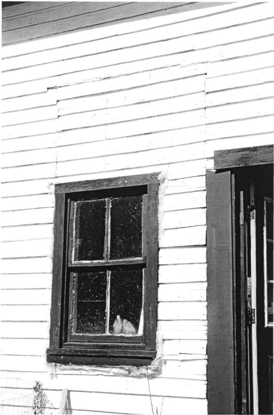
HO-0253 Old Florence School 3055 Florence Road, Southeast elevation-patched opening Ken Short, April 2006 4/9
