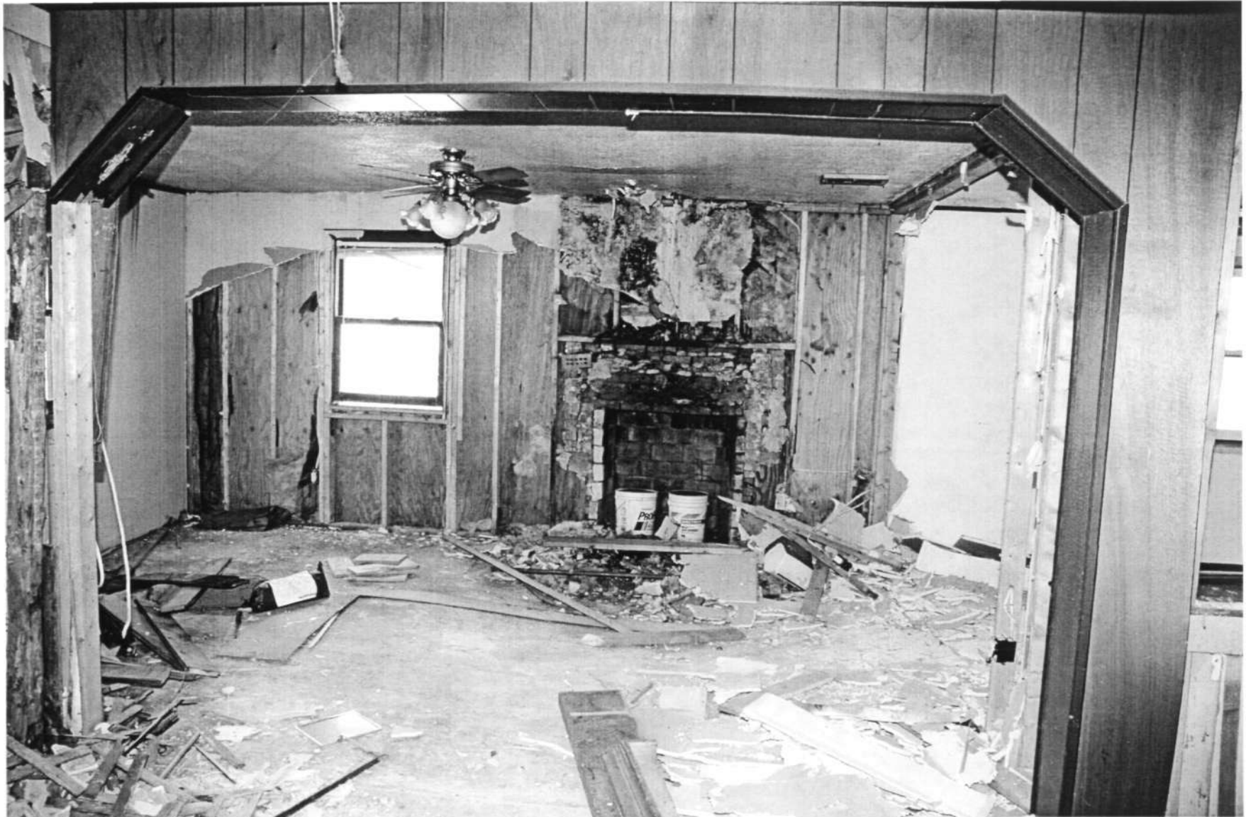
HO-0253 Old Florence School 3055 Florence Road, View northwest into addition Ken Short, April 2006 8/9
