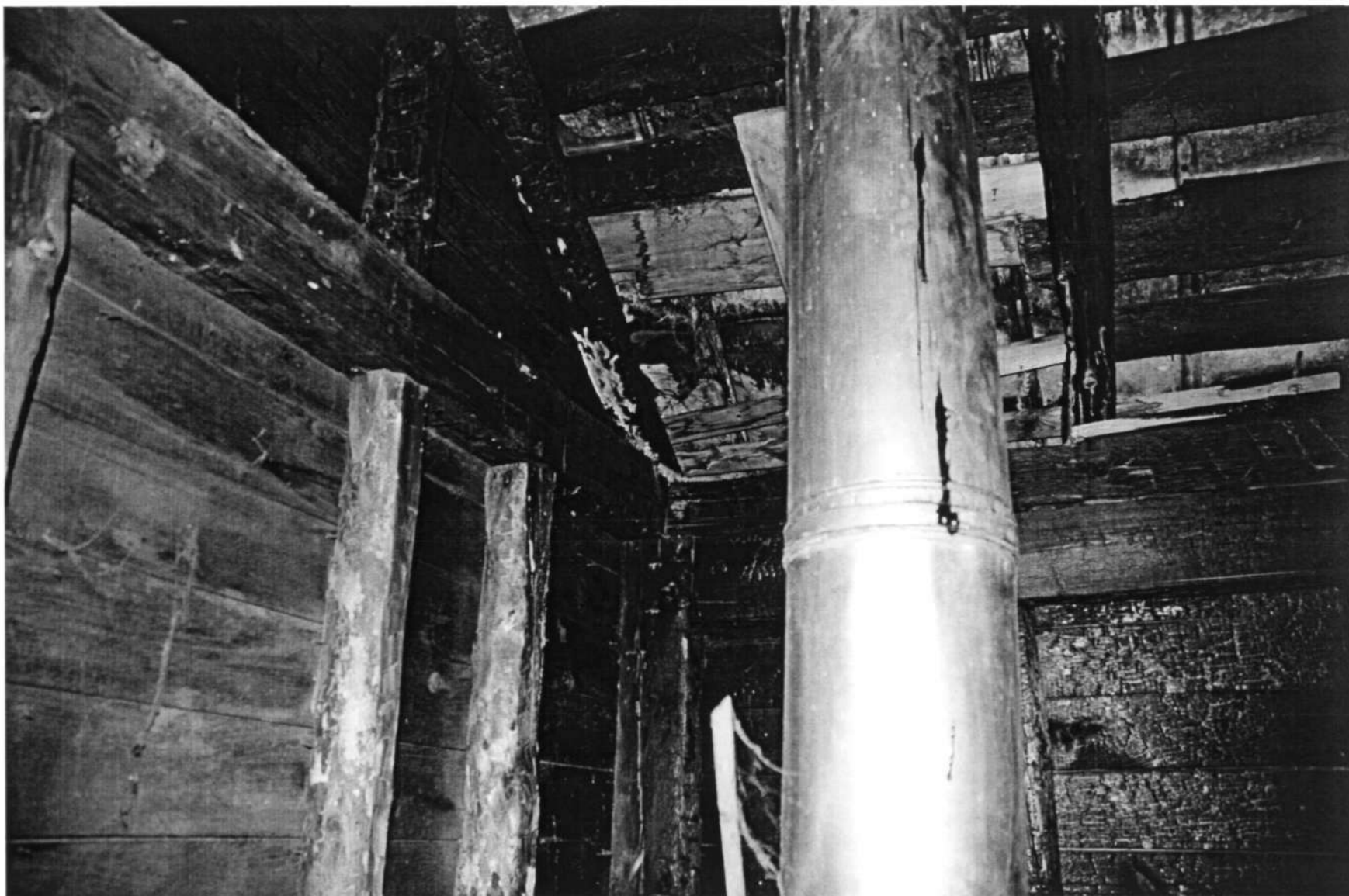
HO-0253 Old Florence School 3055 Florence Road, South corner framing in attic Ken Short, April 2006 9/9
