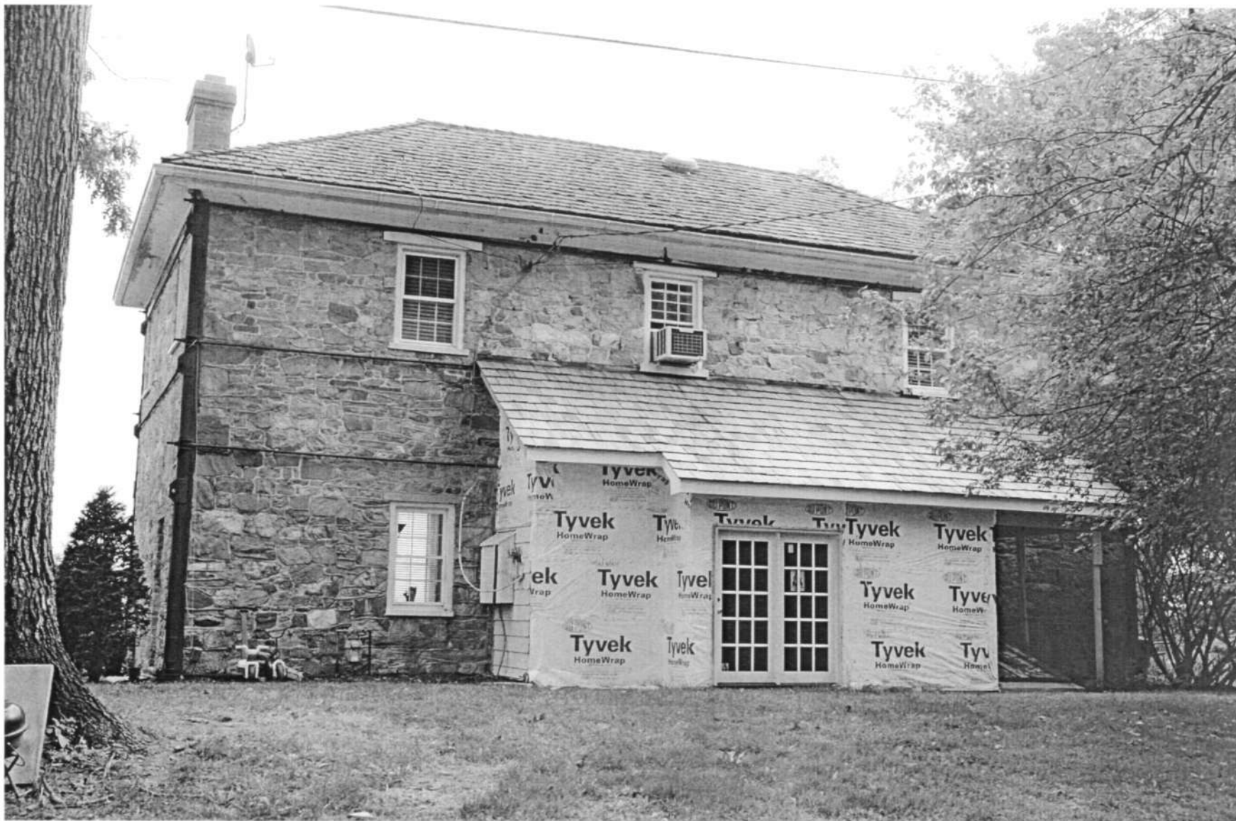
HO-238 "Glenelg" Gardener's House 12789 Folly Quarter Road Northwest elevation Ken Short, September 2006 3/6
