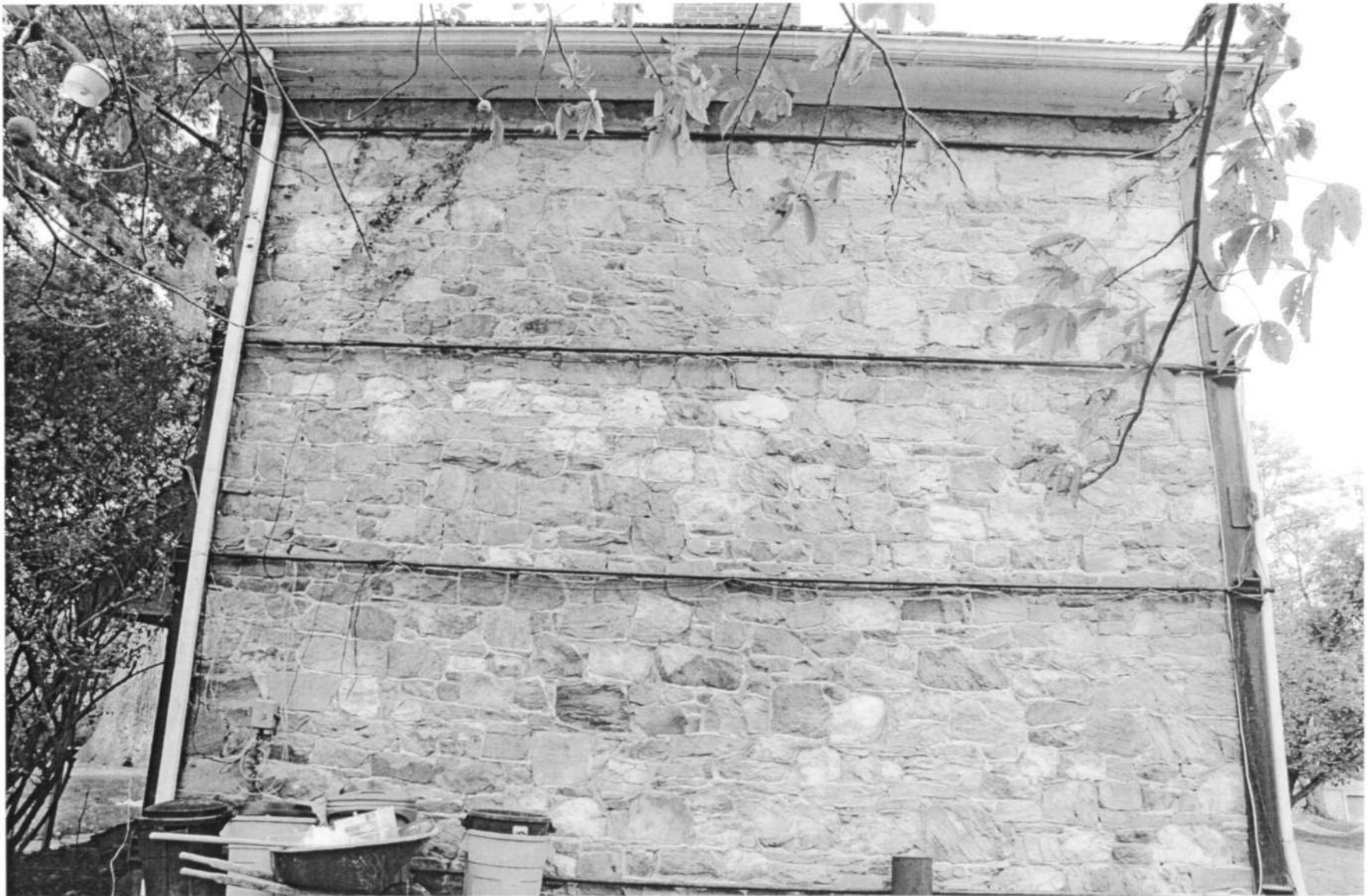
HO-238 "Glenelg" Gardener's House 12789 Folly Quarter Road Southwest elevation Ken Short, September 2006 2/6
