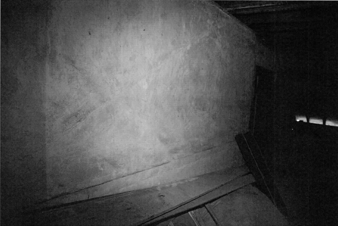
Photo 19 of 20: Hyphen, second story, south wall with ghost of roof pitch and chair rail. 7/11/2018
