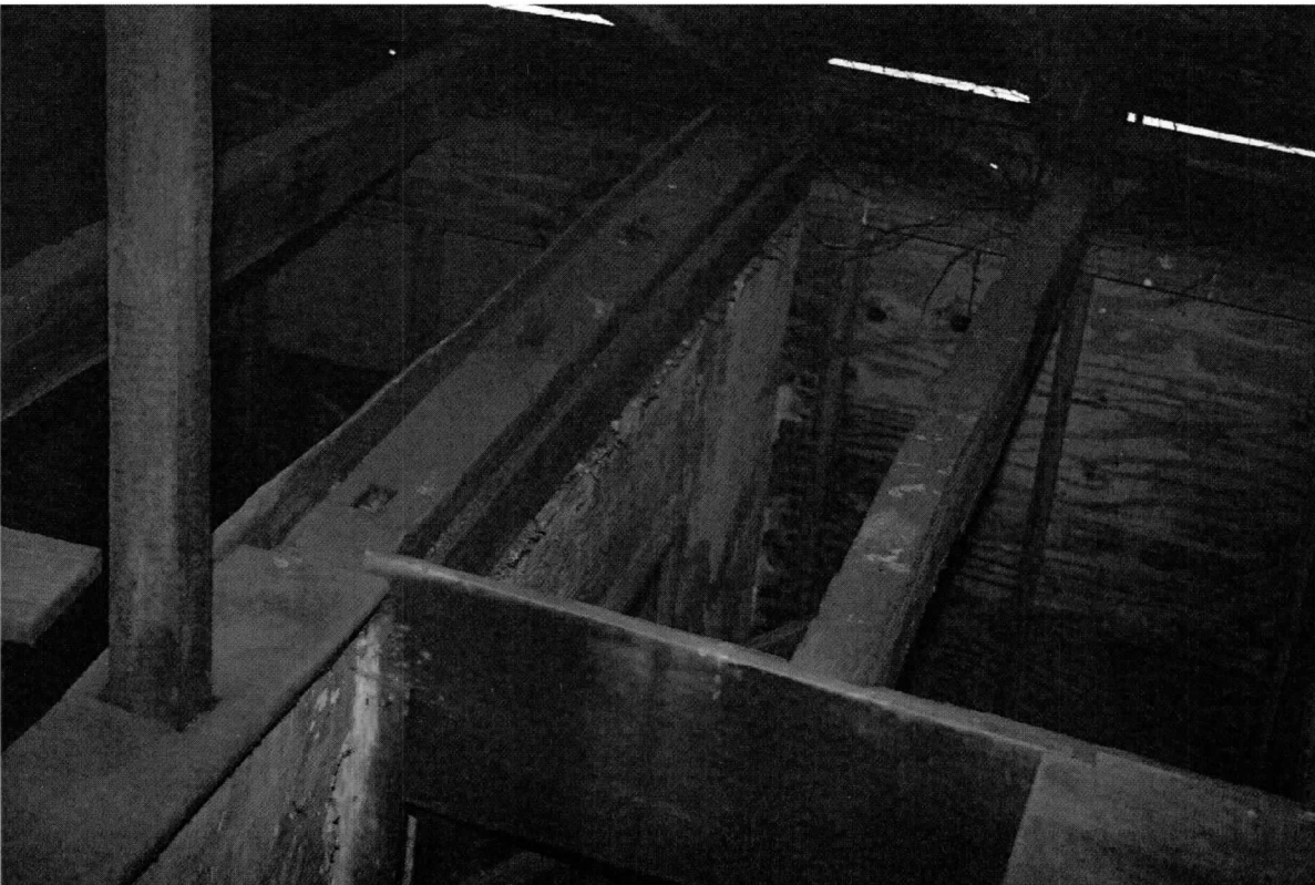
Photo 20 of 20: Top of wall between hyphen and frame section. showing abandoned mortises. 7/11/20
