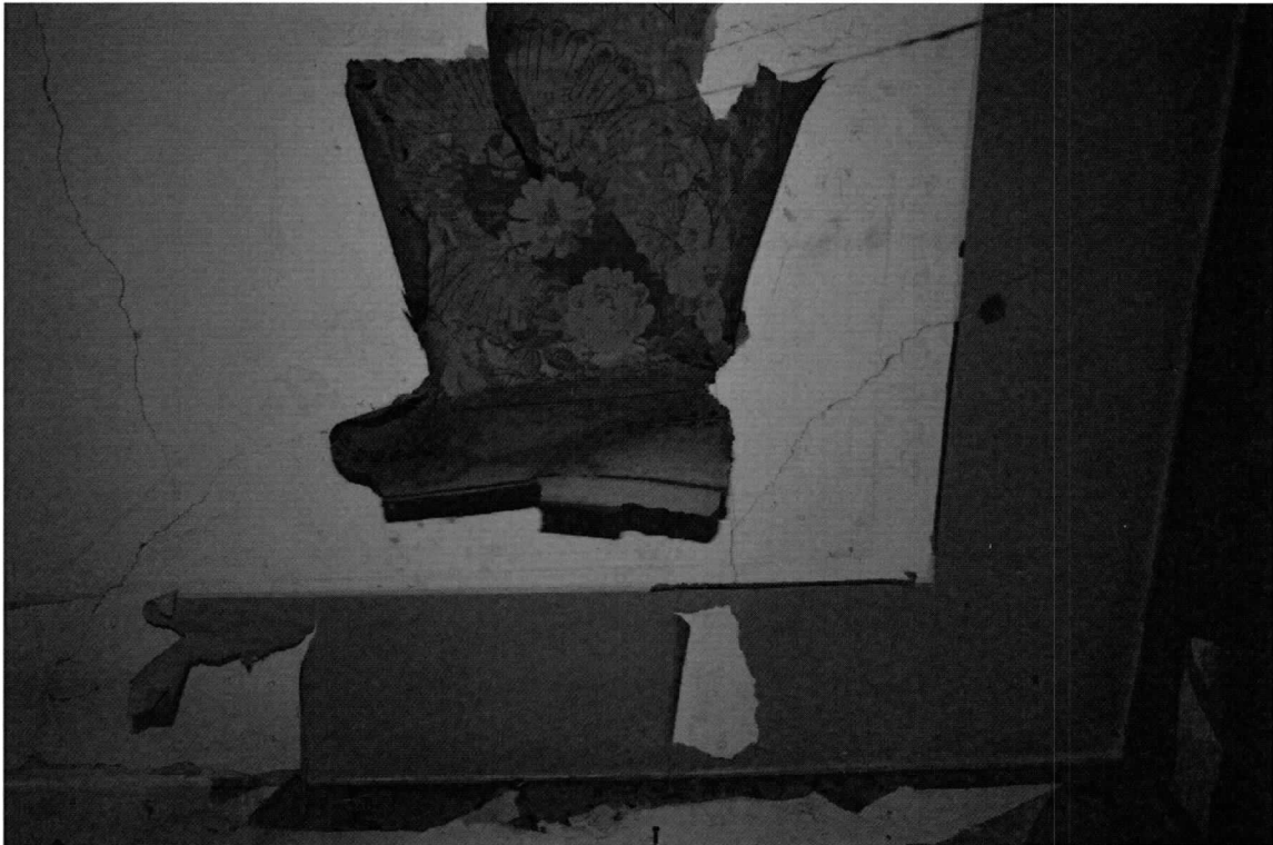
Photo 11 of 24: West room ceiling papers. 3/20/2019
