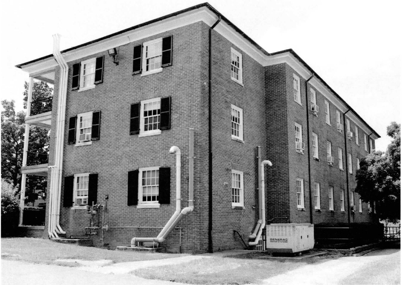
F-3-288 Maryland School for the Deaf Historic District Frederick City, Frederick County, Maryland Meredith Katz August 02, 2021 Building 3; Foxwell-Moylan Hall, east elevation 06/25
