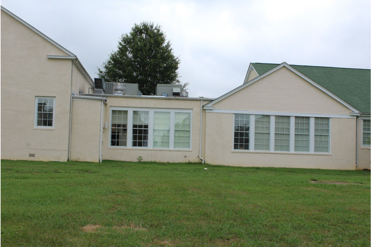
15 of 41 (MD_Charles_BelAltonHighSchool_0015) View Bel Alton High School west elevation looking at north end
